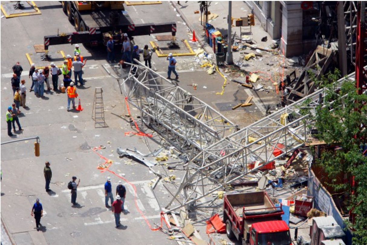
The scene of the crane collapse on the Upper East Side in 2008. Photo: AP
